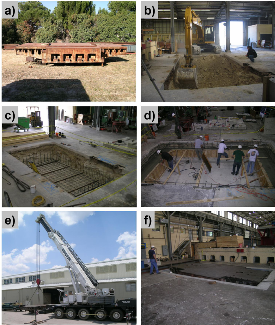
Figure 3-1: a) Platen; b) Excavation; c) Excavated pit; d) Foundation construction; e) Platen lift; f) Platen in position
