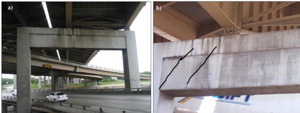
Figure 2-14: a) Interstate 345 pier cap in Dallas, TX; b) Highlighted diagonal shear cracks
